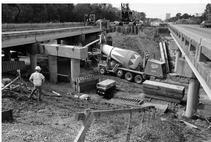
A view from between the I-12 east and westbound travel lanes at 4-H Club Road in Livingston Parish
